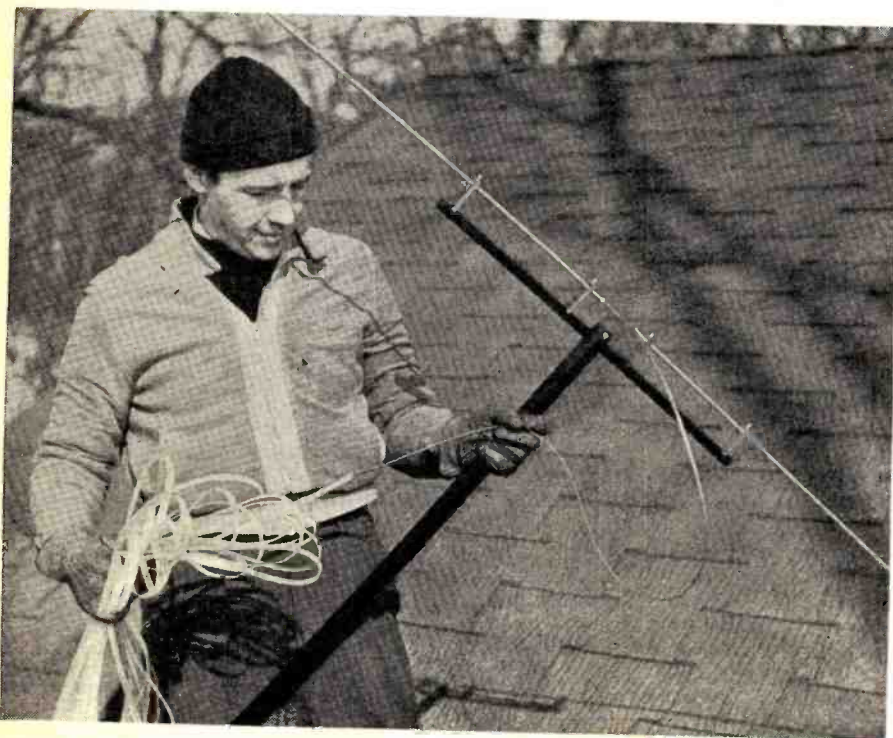
Fig. 7. Assembled dipole with lead-in and matching section attached ready for installation. Television technician shown is Jack McNally.
